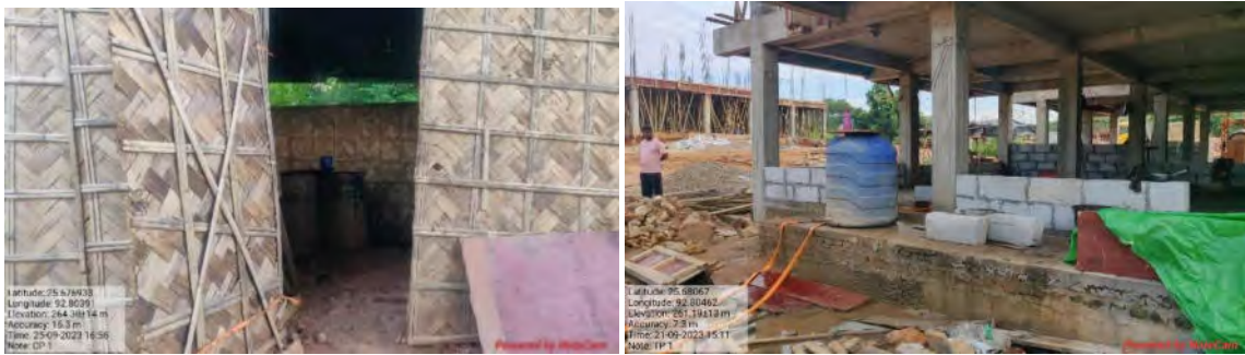
Unsafe drinking water at CP1
