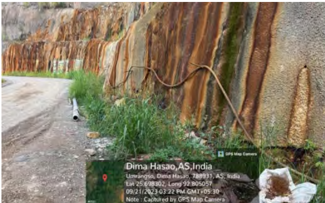
Kopili Seepage water near the Tail Race Tunnel and Power House.
