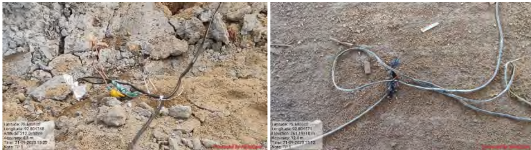
Lose wires at CP 1 construction site
