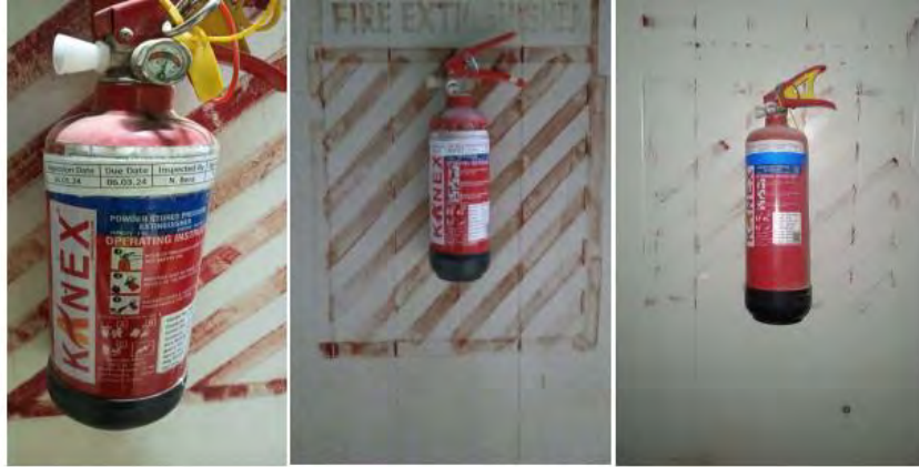
Fire extinguisher inspection CP-2
