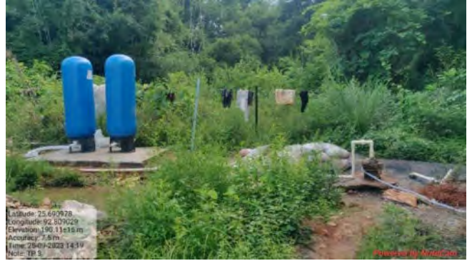
RO facility installed at CP3
