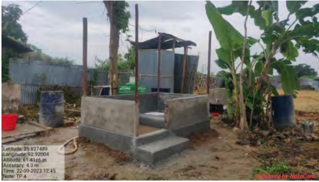
Toilet facility at CP4 storage yard
