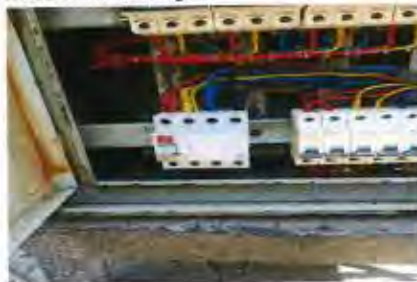
RCCB is not working.
